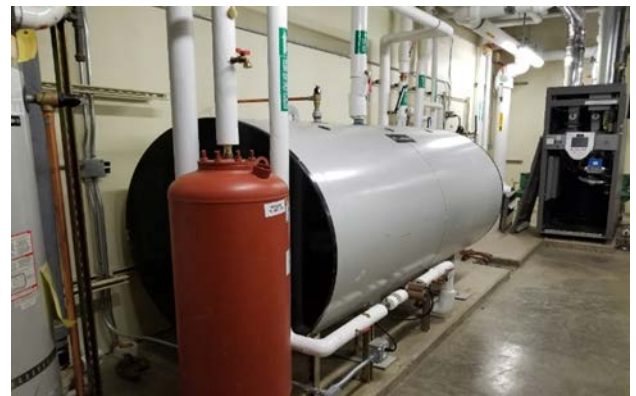
Boiler at Blackfeet Dormitory in Montana
